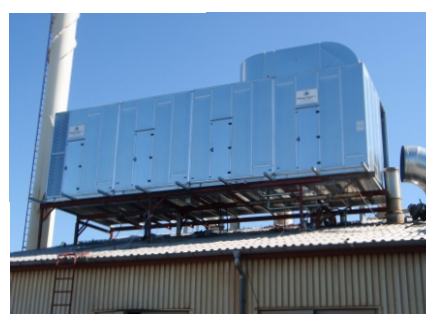
Offshoreindustri: Danbor, Esbjerg Ventilation, 60.000 m³/h
